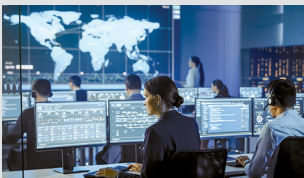
Automated Logic developed the basis of design for the BMS at Iron Mountain Data Centers.
